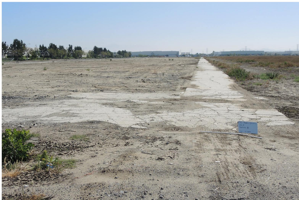
Plate 5.2.1-16: Overview of Feature B feed alley foundation remnants at Site CA-SBR-33,113H, facing east.
