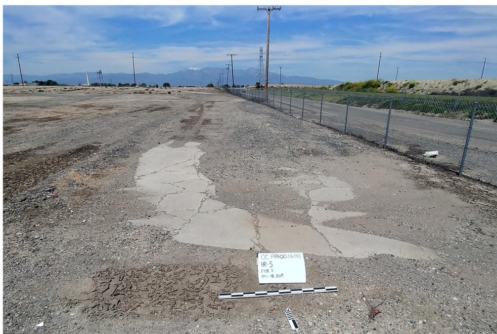
Plate 5.2.4-7: Overview of the Feature F concrete driveway at Site CA-SBR-33,116H, facing north.
