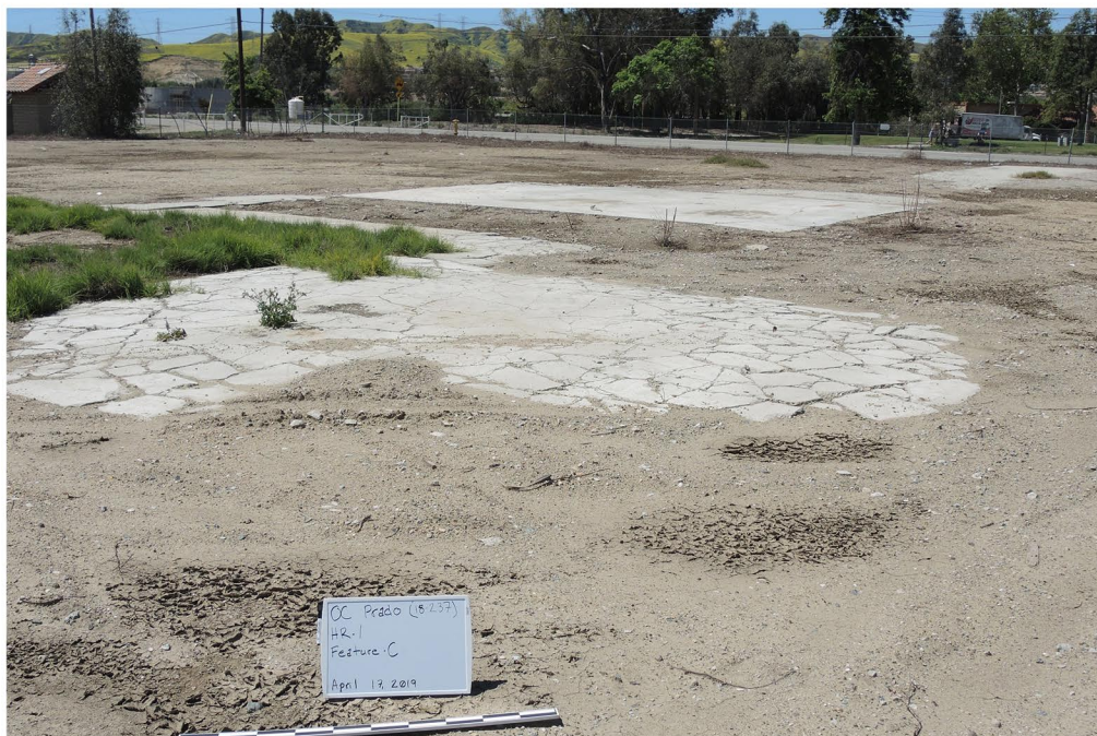
Plate 5.2.1-3: Overview of 1955 Feature C residence and garage foundation remnants at Site CA-SBR-33,112H, facing southwest.
