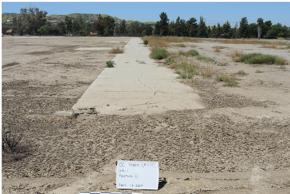
Plate 5.2.1-2: Overview of 1955 Feature B dairy structure foundation remnants at Site CA-SBR-33,112H, facing west.
