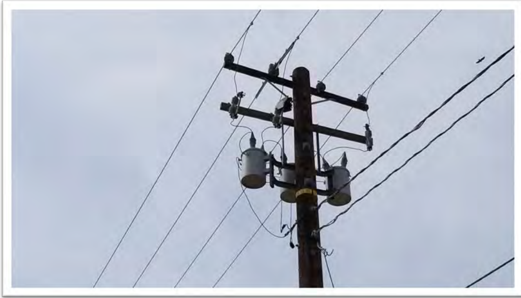
Photo 11. North-South Trending Electrical Power Lines in Eastern Portion of the Property.
