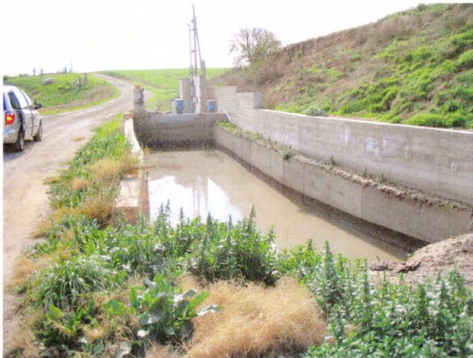
Overview of sump near Arthur residence where discharge water from 18" concrete line drains and is then pumped up to holding pond.
