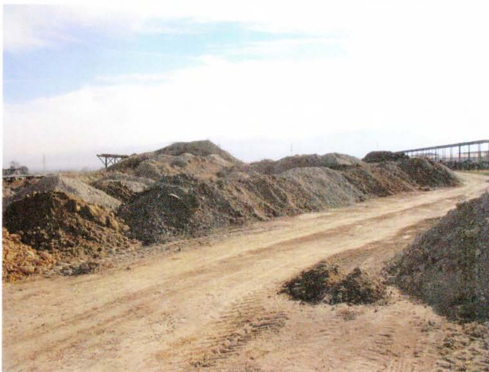
Soil stockpiles at northwest portion of property.
