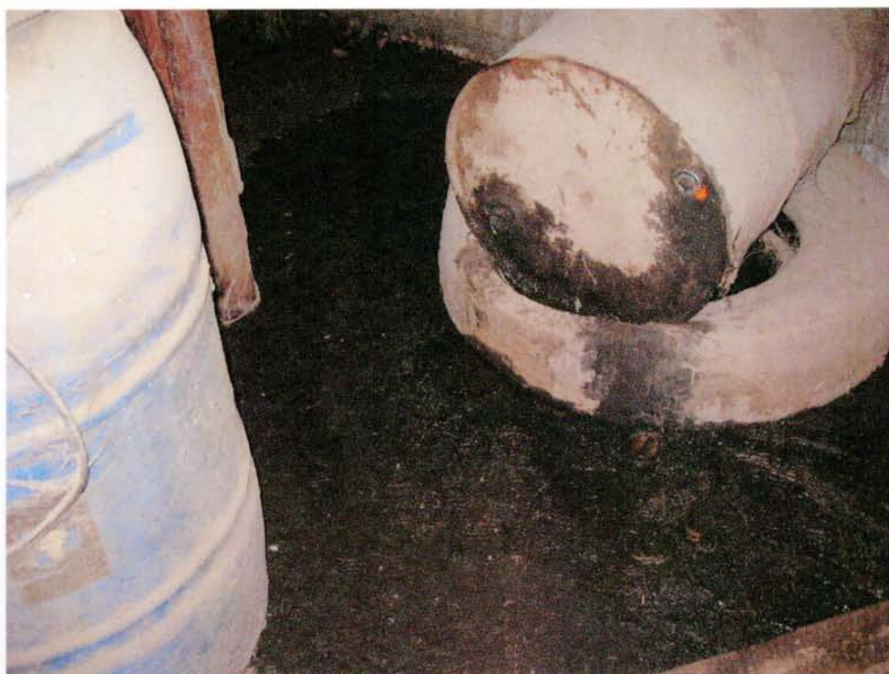
Surficial staining on concrete beneath leaking 55-gallon drum in maintenance shed near milking barn.
