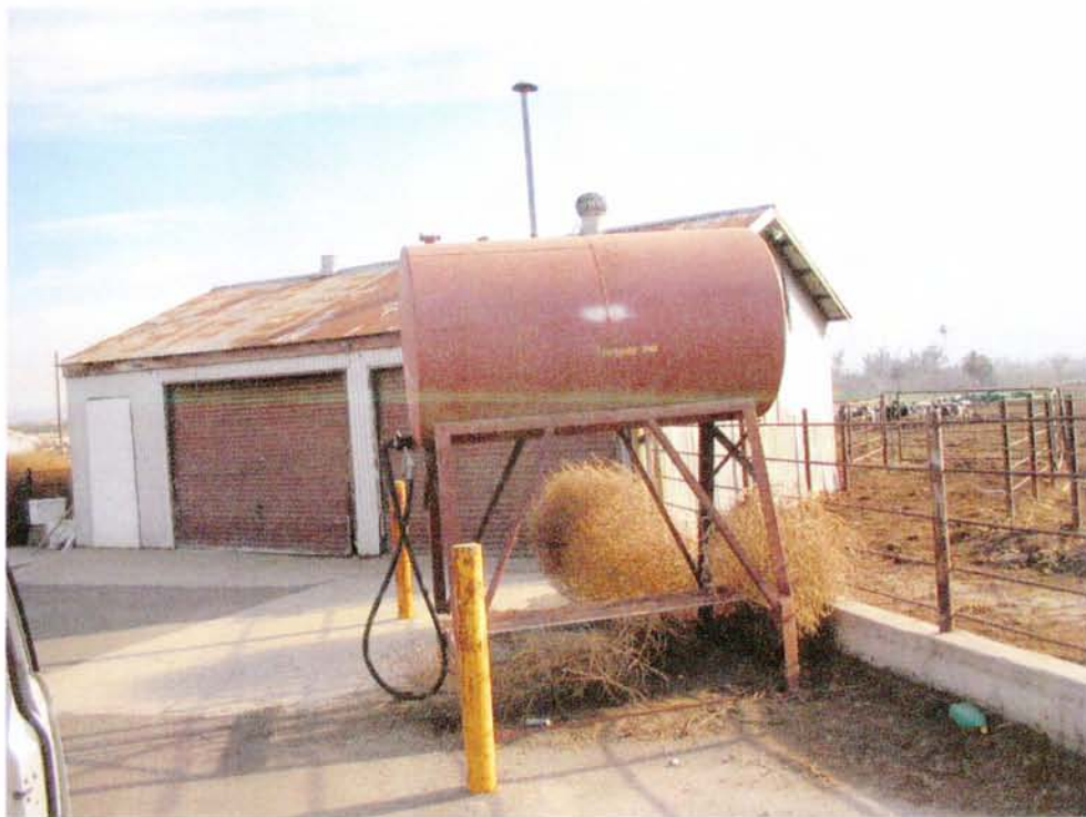
500-gallon unleaded gasoline AST at residence.
