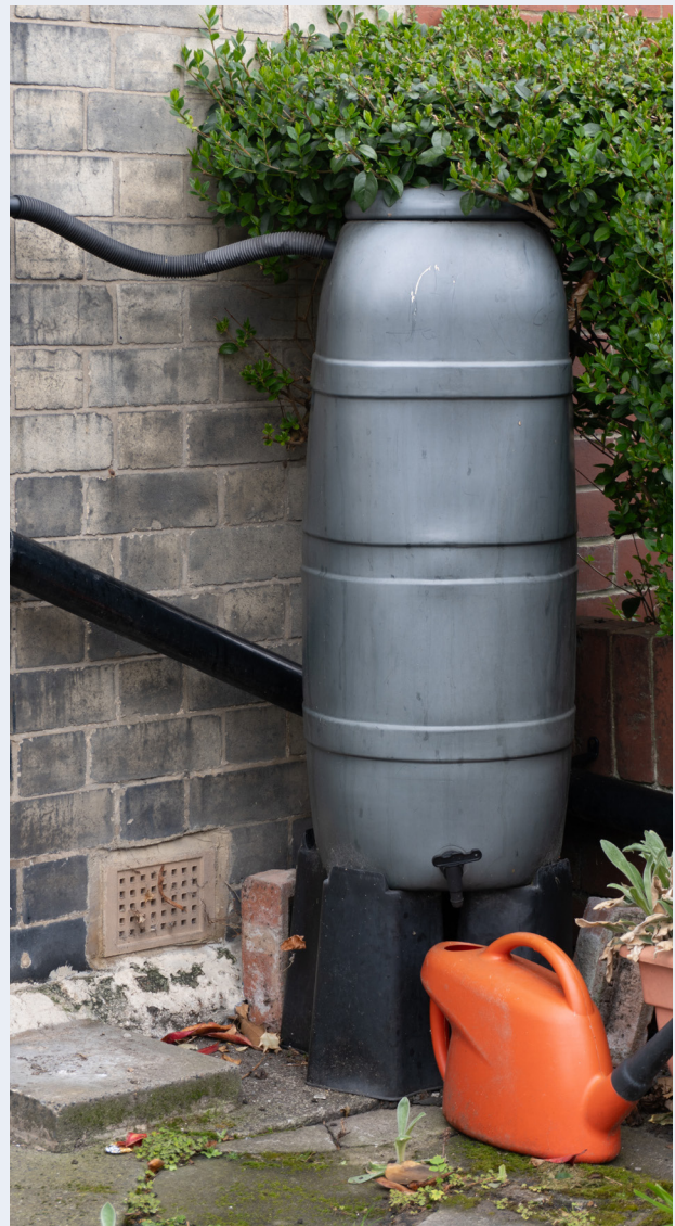
Rainwater harvesting system
