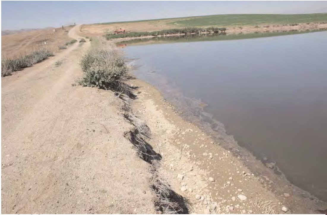
PHOTOGRAPH 5: Agricultural pond created by excavating and/or diking dry land. Note prominent berm that separates agricultural pond from Mill or Chino Creek and maintains hydrologic separation. Pond is maintained and generally supports little or no vegetation as shown.
