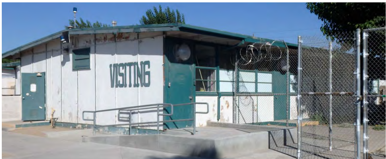
Visiting building with peeling paint.
