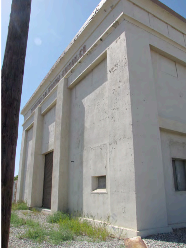
View westerly of the front (south) elevation, showing first floor fenestration alterations and painted-over second-story and frieze windows. The original dimensions for the first floor windows and door openings are still visible.
