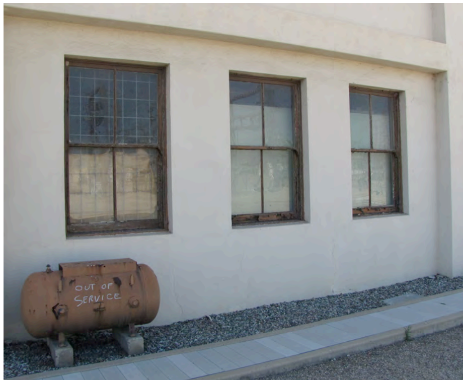
Typical historic two-over-two wood windows punched into the façade, with a cable raceway (trench) in the foreground.
