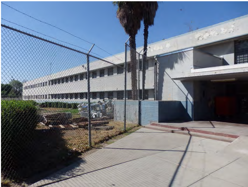
South end of building. Projecting cornice and balcony do not extend over northern-most 85 feet.
