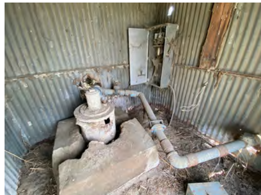
18. Well shed wellhead
