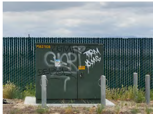
30. Typical adjoining transformer
